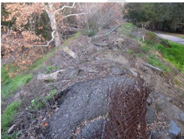
Photograph 7. Debris between trail and creek.
