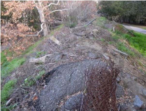
Photograph 7. Debris between trail and creek.
