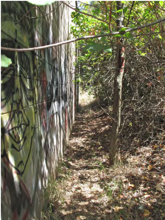
Pinch point downstream of Mockingbird Lane.
