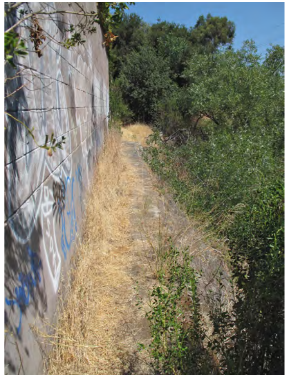
Pinch point near Permanente Creek Bypass.
