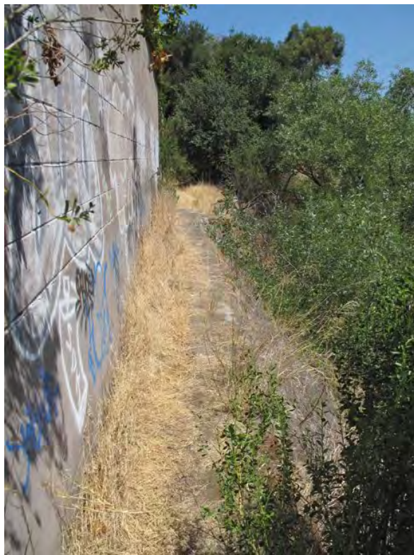
Inadequate top-of-bank behind the soundwall along State Route 85 at a channel meander.
