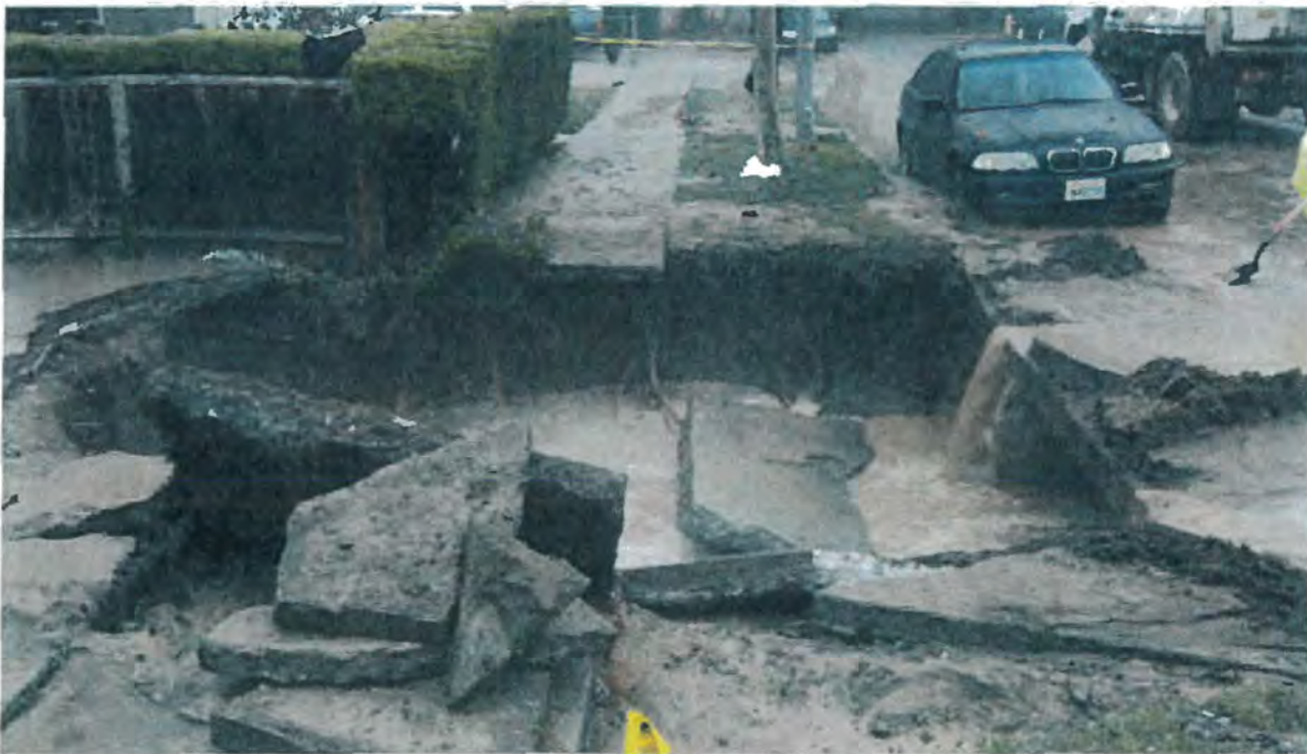
Figure 1. Damage observed due to main break located on Pensacola Drive in the eastern side of San Jose.
