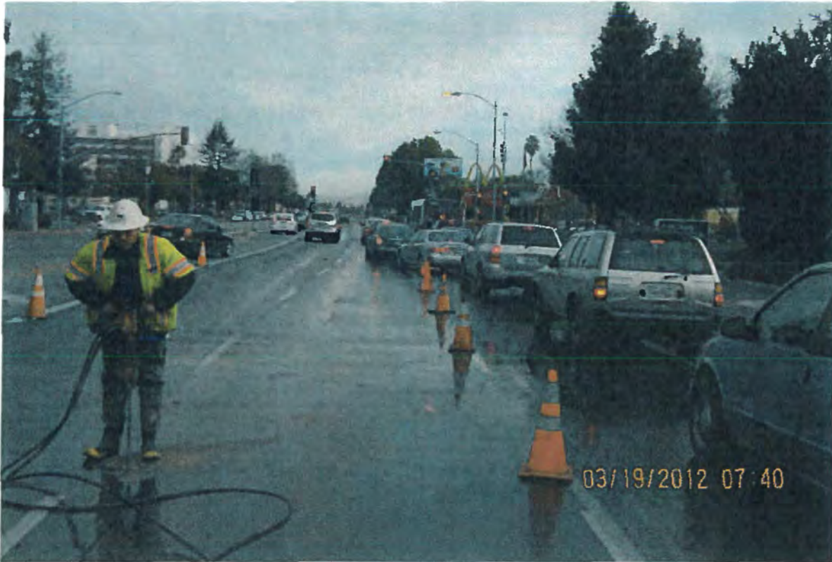
Figure 2. Workers diverting traffic on Bascom Avenue while attempting to fix a main break on a 12" water main.
