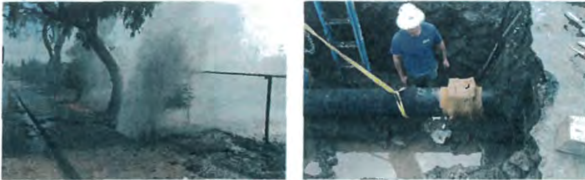
Figure 3. Picture on the left illustrates the Break Stage of a main break; picture on the right illustrates a repair during the Isolation Stage of a main break.
