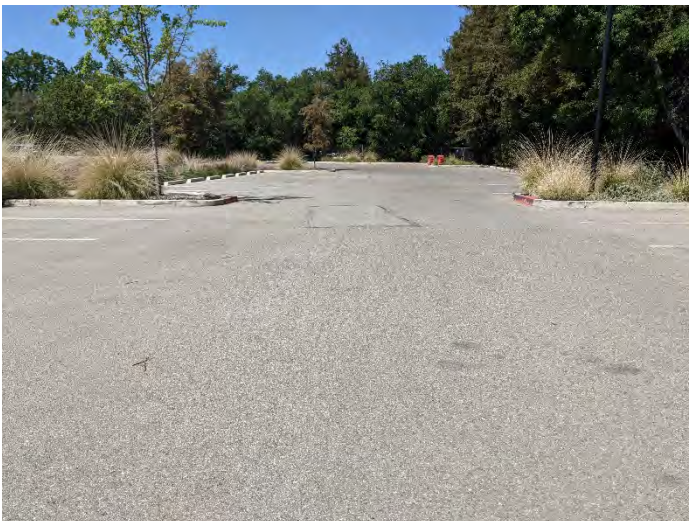
Photo 17: View of rectangular asphalt patch in northernmost portion of parking lot, looking northwest.
