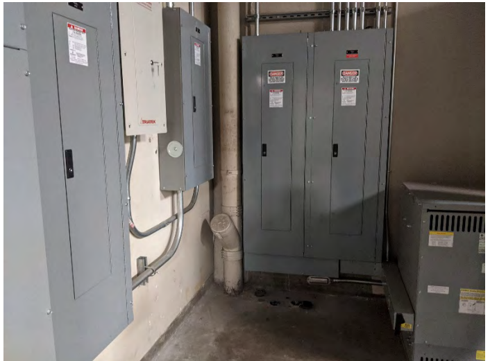
Photo 10: View of electrical fuse closets in northeast portion of Subject Property building.
