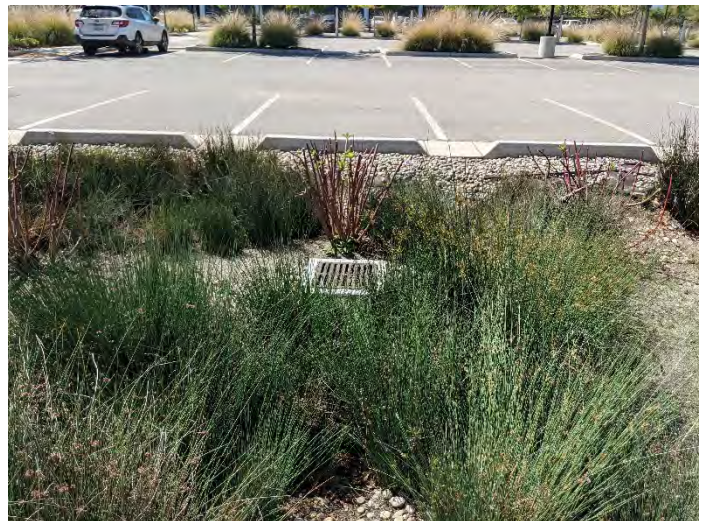
Photo 16: View of typical storm water drainage system in north parking lot.
