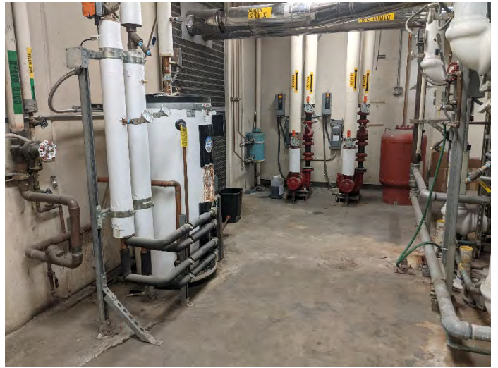
Photo 8: View of water heater and hot water lines in northeast portion of Subject Property building.
