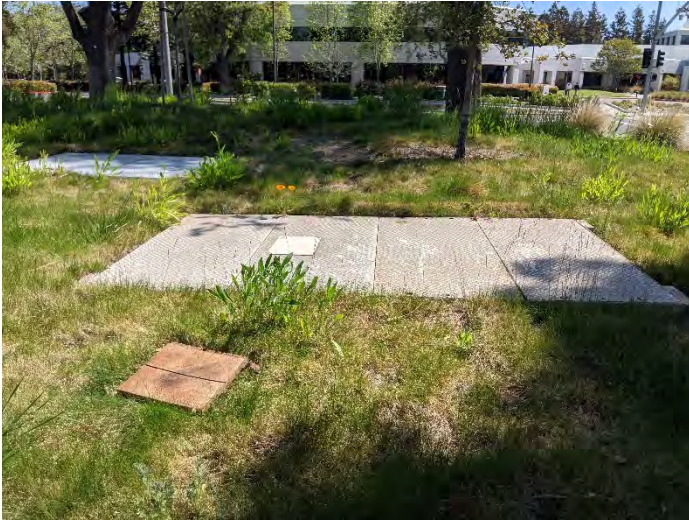
Photo 13: Utility boxes in landscaping near southeast corner of Subject Property.
