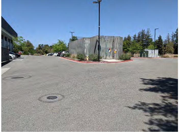
Photo 14: View of utility enclosure with cooling units and diesel generator; pad mounted transformer to right.
