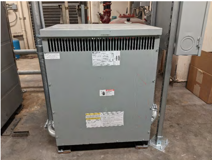
Photo 9: View of dry-type transformer in northeast portion of Subject Property building.
