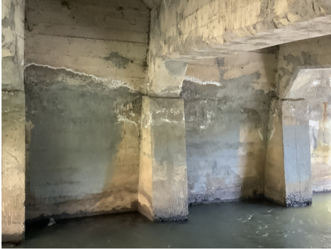
Photo 3 Patched areas on Abutment 2
