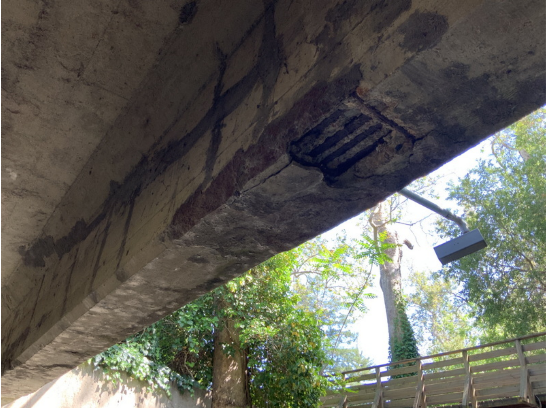
Photo #2 Spall with exposed rebar in the bottom of Girder 6
