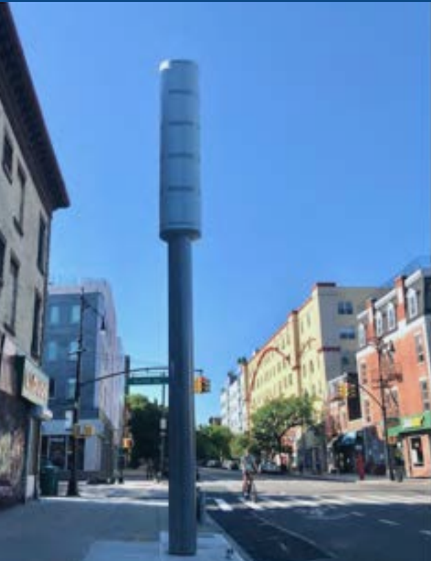
New York City Jumbo 5G poles with 5 tiers to house transmitting antennas from numerous carriers.
