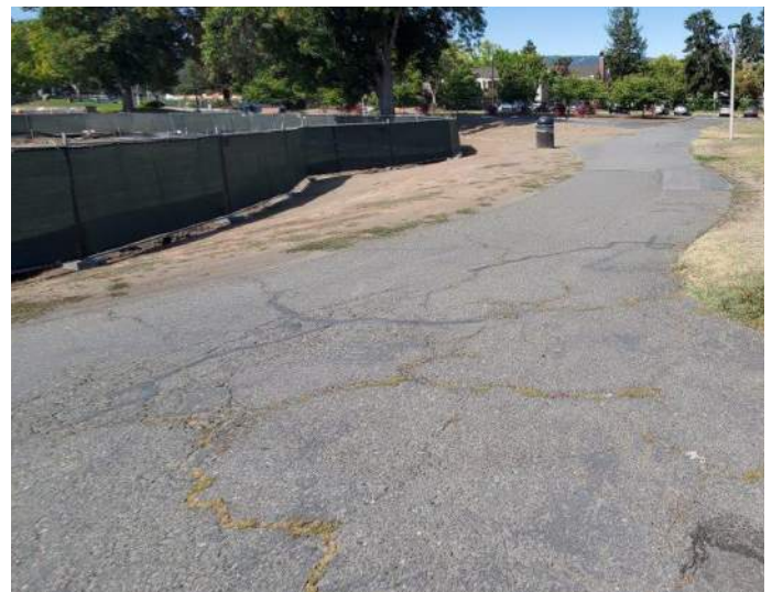
Image 2-7: Cracked Asphalt Path
