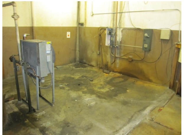
Photograph 20. Staining on floor near drain at former compressor location in basement at SAC.
