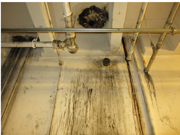
Photograph 21. Waste oil drain in floor slab, capped drain pipe in wall and wall staining in basement at SAC.
