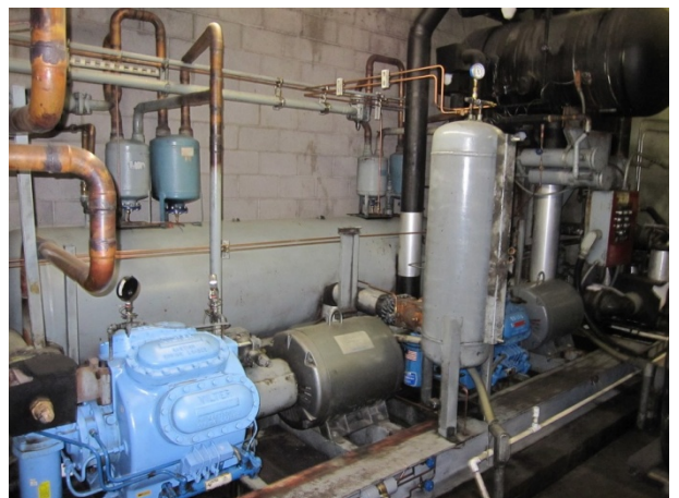
Photograph 8. Refrigeration equipment at Cupertino Ice Center.
