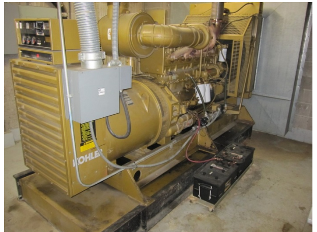
Photograph 6. One of three on-site emergency generators.
