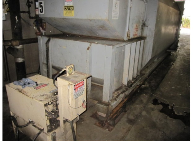
Photograph 12. Typical trash compactor and associated hydraulic fluid AST.
