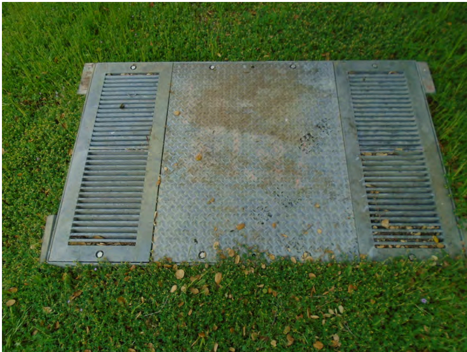
8. View of subsurface transformer on subject property
